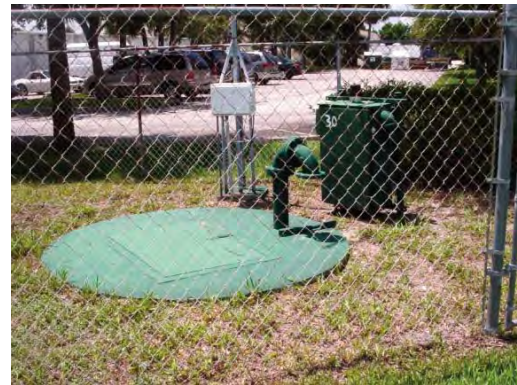
Lift Station Odor and Airborne Bacteria control
